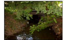
Ref 14 6/RN/As/SLB.50) Outlet of concrete box culvert at Drummond Road. Size: 1.880 x 0.760.
